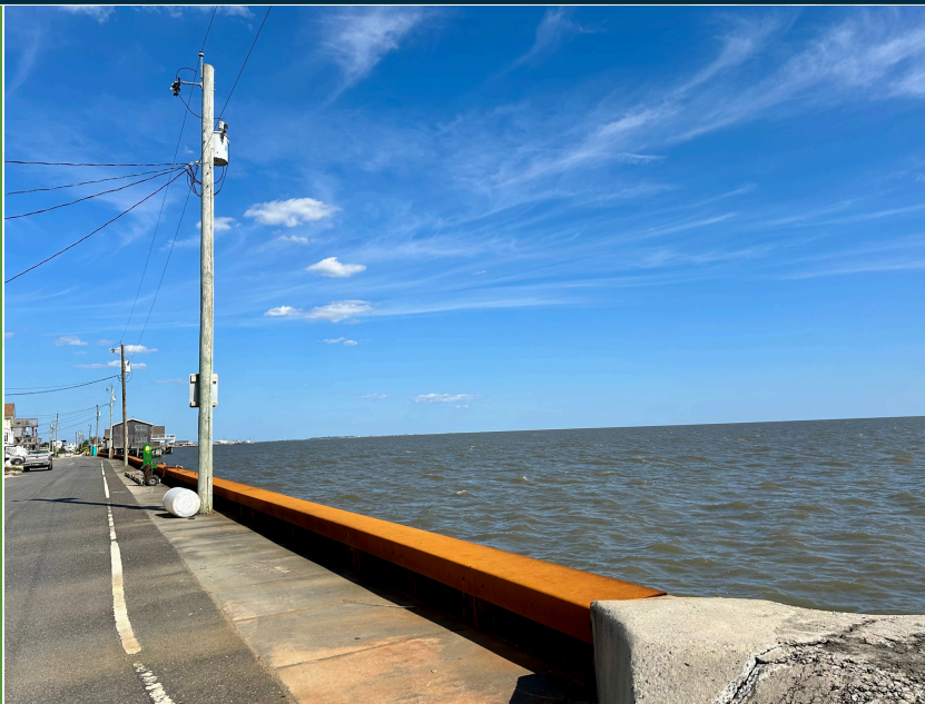
A Breath Taking View from Gandy's Beach. This photo of the Bulkhead Repair Project was taken as the Project was nearing completion.
